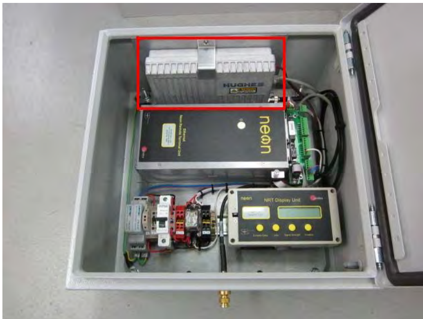
Locate the Hughes modem in the system. Shown with red box
